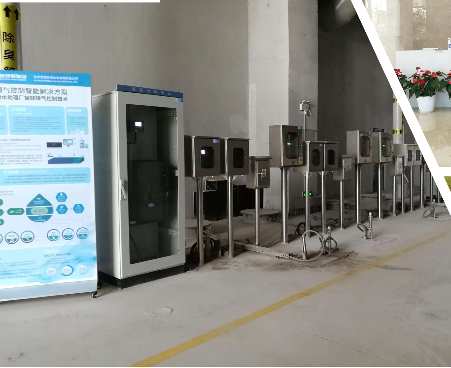
Beijing Capital, Dongba WWTP
